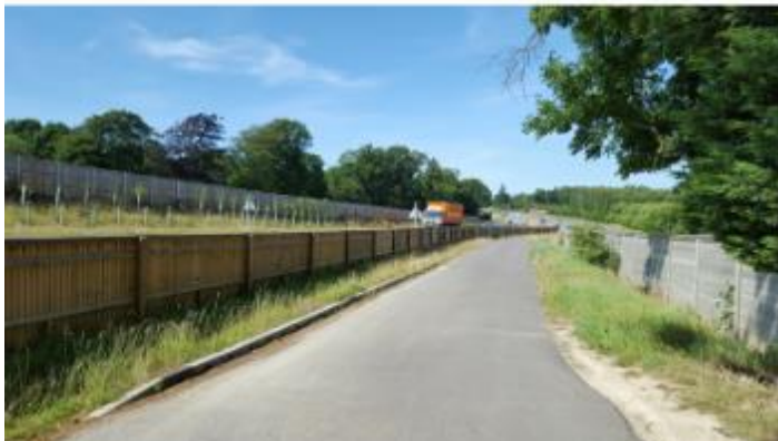
Environmental (noise) barriers and segregation from the southbound carriage of the A21 at Yew Tree Farmhouse
