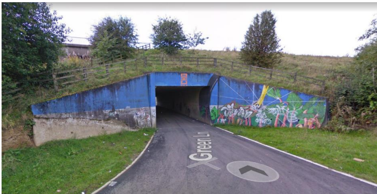
Figure 5.7 Horbury Underpass / Green Lane viewed from the east (source: Google Streetview, August 2020)
