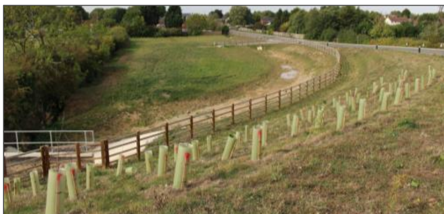
Figure 25 View from Town Street bridge towards South Killingholme illustrating failed plants marked up for replacement, shelters not maintained upright and several not fixed in position.
