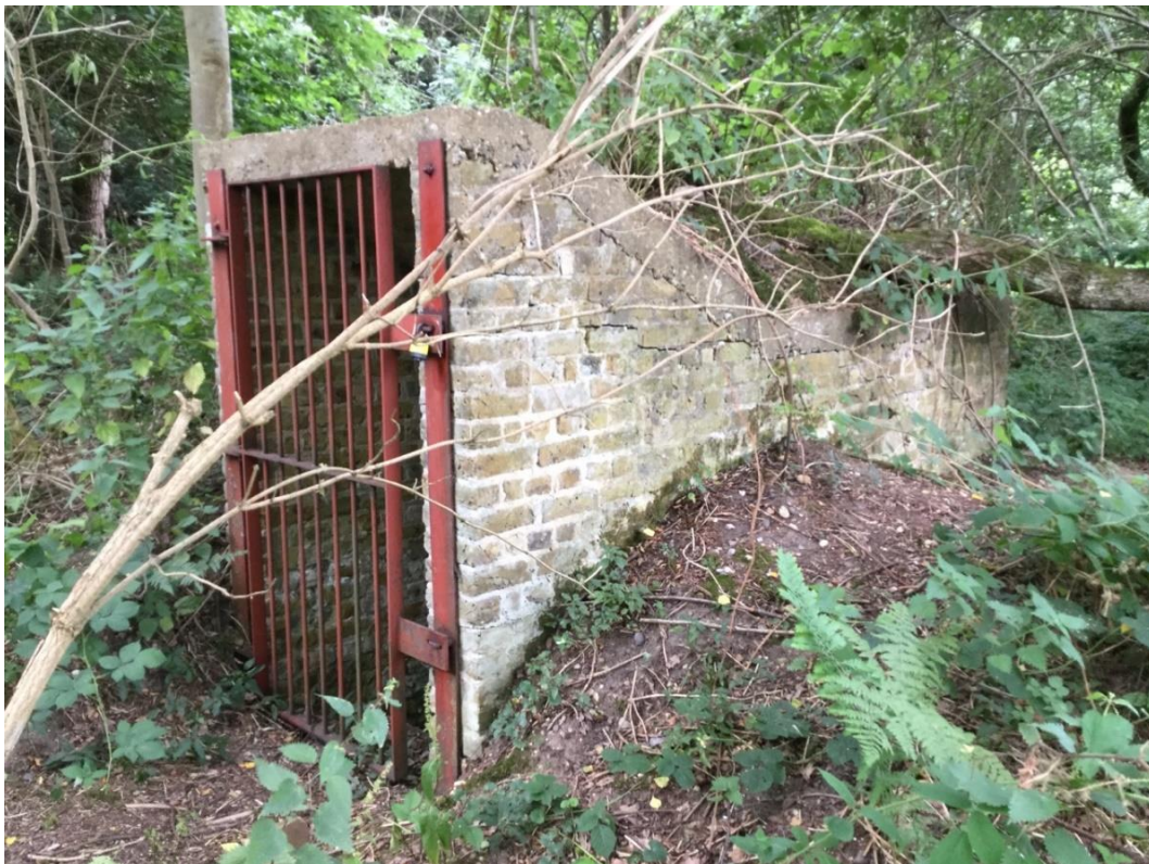
Plate B.85 Standing structure associated with Ashenbank RAF Camp, likely air raid shelter (1842), image looking south-west
