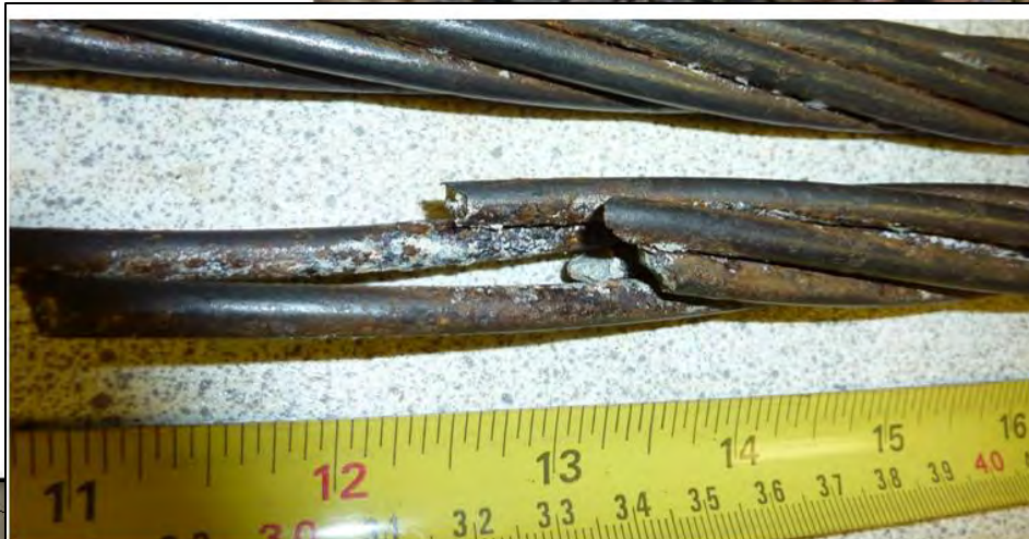
Fractured Wires on Tendon #1
