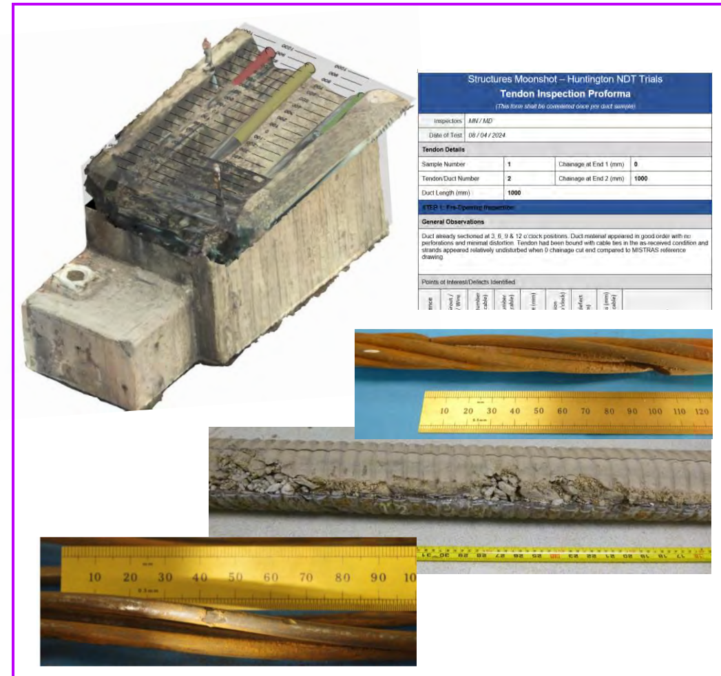
Actual defects recorded during hydrodemolition and intrusive inspection
