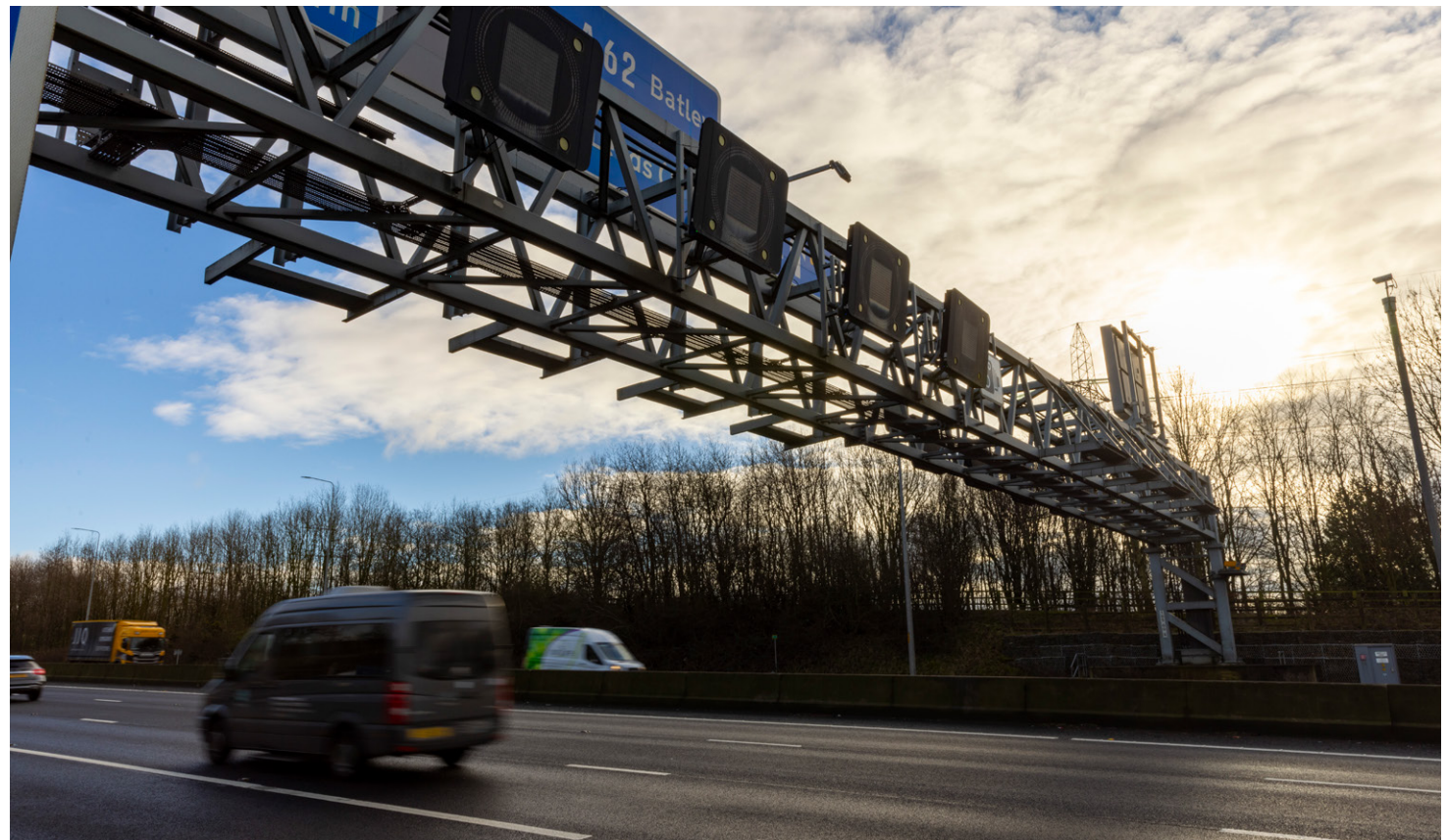
Sign and signal gantry on the M62 DHS motorway
