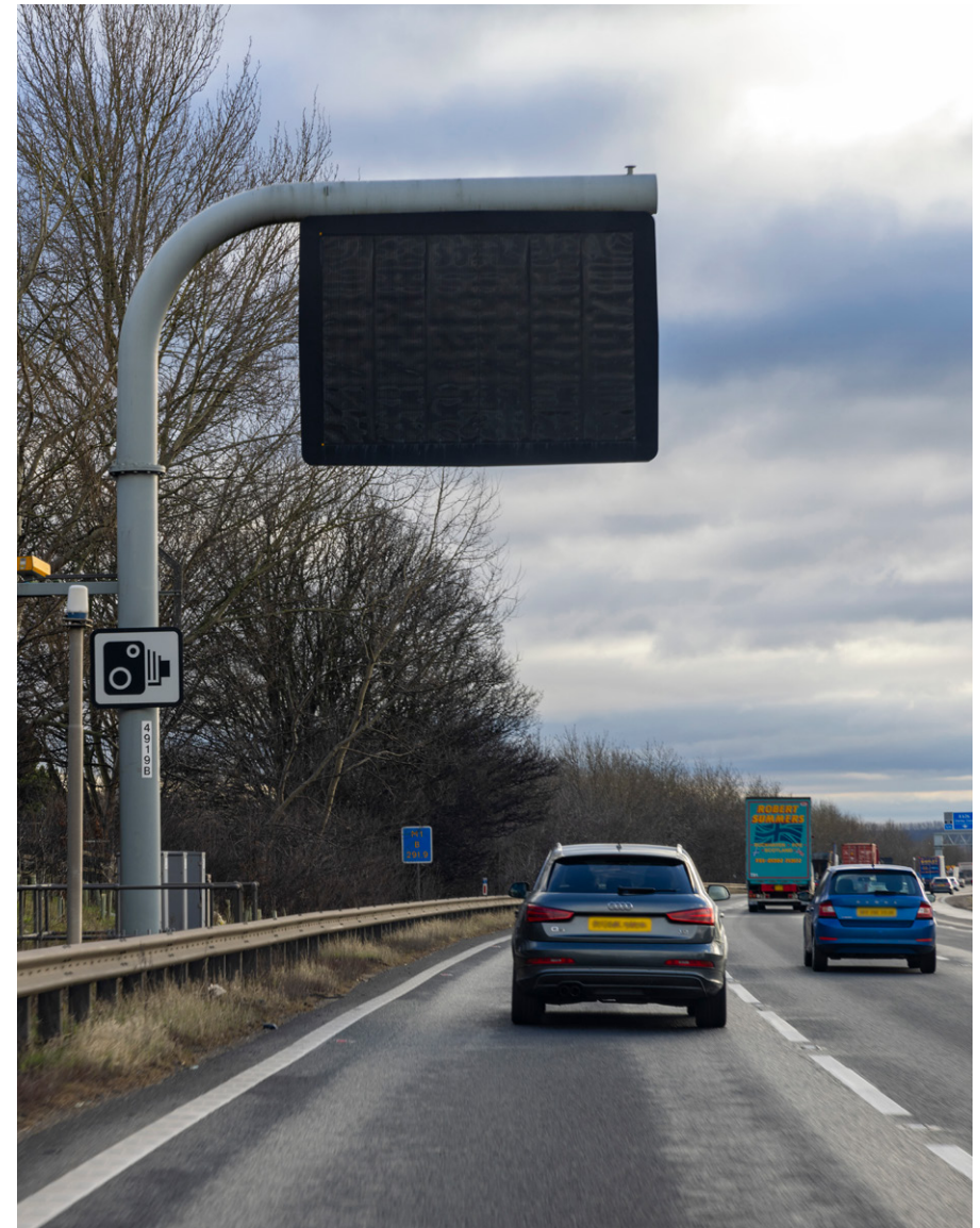
Smart motorway technology
