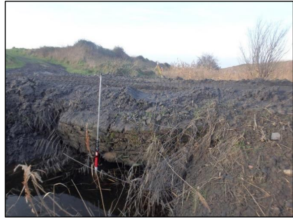
View 2: Upstream view of culvert crossing to the east of the Project road.
