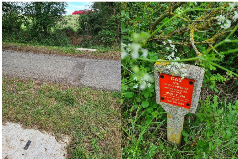
Indicative condition of roads between industrial sites to the south of the nitrogen deposition compensation site. Gas pipeline marker and indications of buried services across Codham Hall Lane to the south of site
