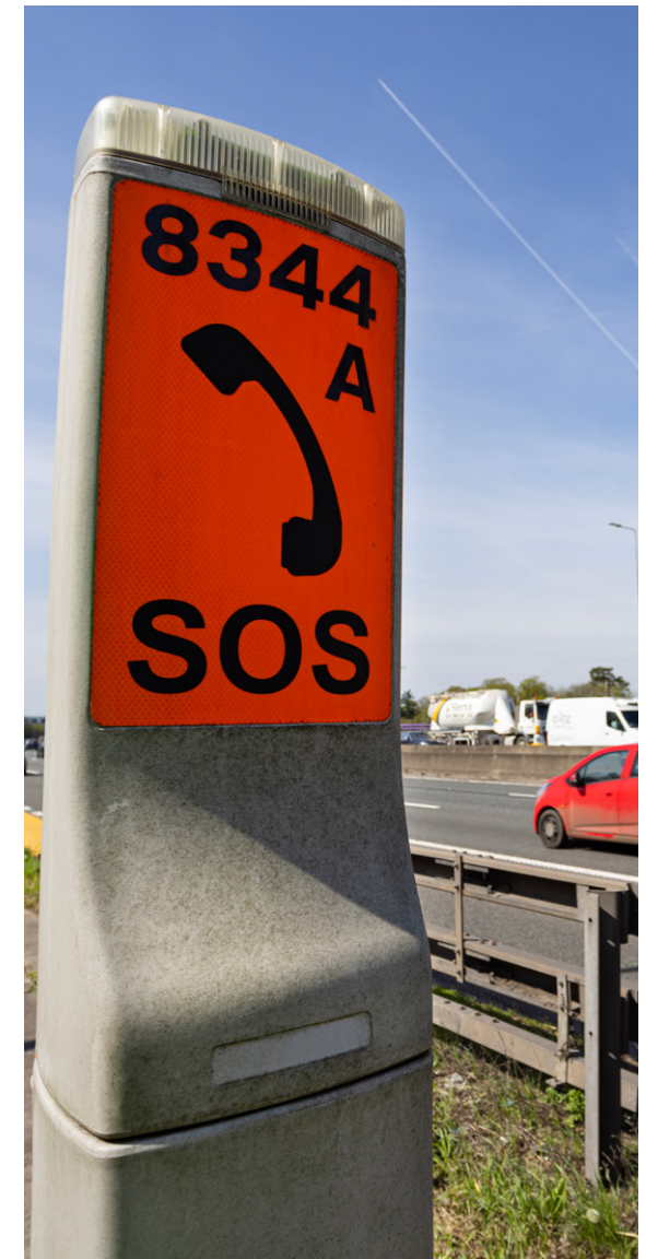
Emergency roadside telephone
