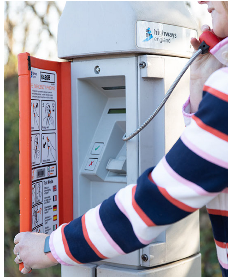
Emergency roadside telephone in use
