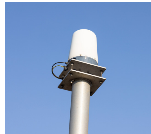
A stopped vehicle detection radar pole
