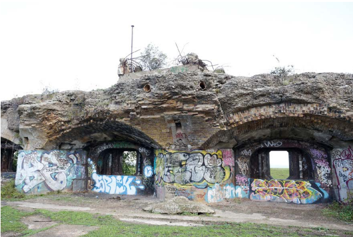
Plate SF4: View of the gun emplacements and construction layers of the casemate. The concrete rubble in the centre hides a lift shaft to the magazines below. The remains of the WWII command post and mine watchers post is visible on the roof.
