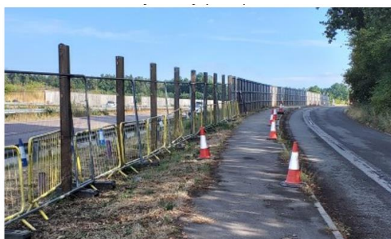
At 5YA barrier was being upgraded with concrete poles (Source: 5YA Evaluation visit August, 2022)
